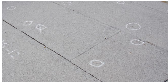
Hail can displace the granules or fracture the underlying reinforcement of the modified bitumen.
