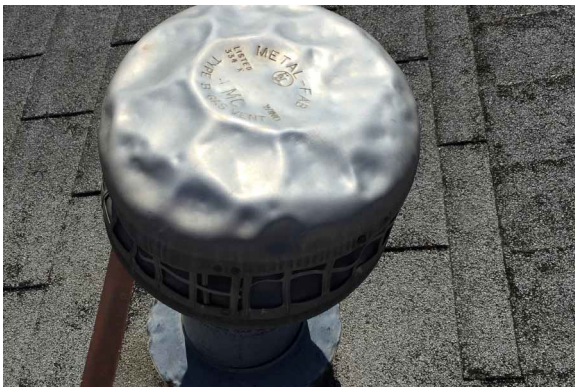
Roof vents that are dented point to signs the roof has sustained damage.
