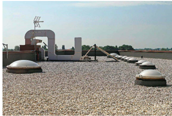
On tar and gravel roofs, the pea gravel must be kept even on the roof at all times. High winds can cause the gravel to move and pile up. Check for cracking or blistering that can lead to failure.
