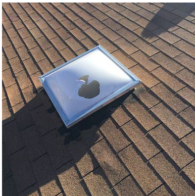
Skylights and window damaged by hail can resemble this image.
