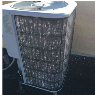
HVAC units can sustain damage to the condenser fins.
