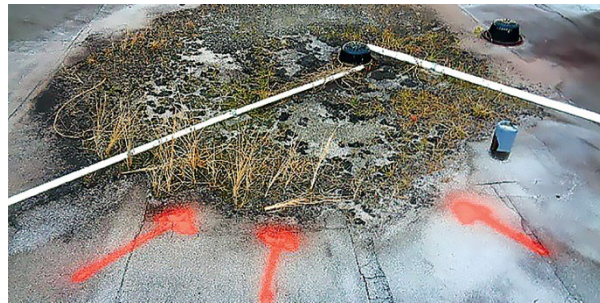
The modified bitumen roof has cracks or fractures where water can accumulate underneath the surface and pool. This excessive moisture can result in plant growth.
