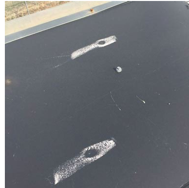
Lay chalk flat on the surface and rub up and down to find hail dings on a metal roof.
